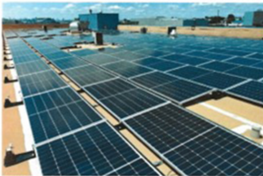
Crystal's New York factory operates with more than 2,300 solar panels that generate one million kW-h annually.
